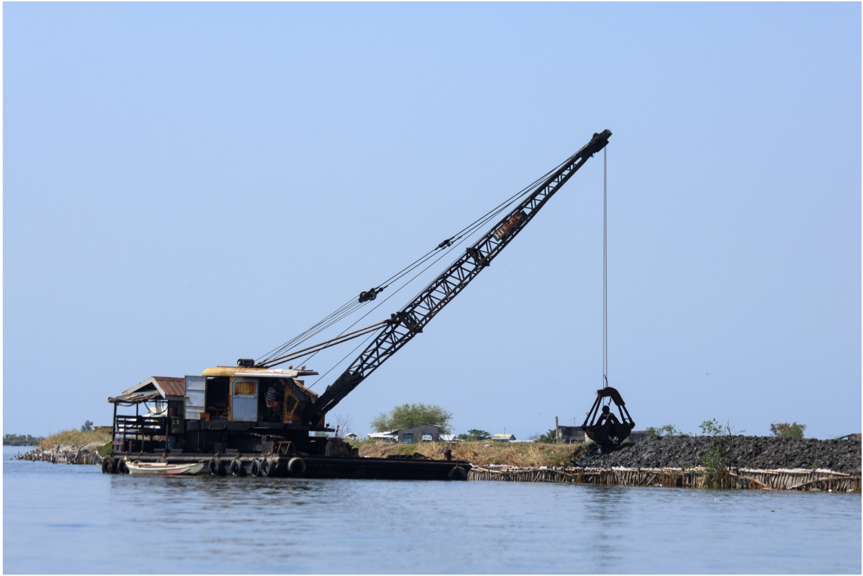
There are dredging stations along the 80.61-kilometer stretch of the Pasac-Guagua Watershed to regularly manage the sediments/lahar from the upstream.
