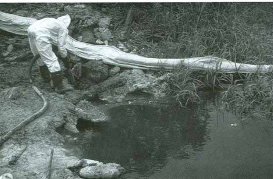
Powell Duffryn chemical storage tank incident, Savannah, Georgia, April 1995. Cleanup workers vacuum chemicals from rocks on the bank of the drainage ditch near the facility.
