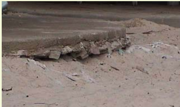
Erosion necessitated the use of sand bags that render the spot unsightly.
