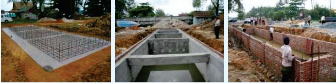
Photos 16–18. In 2011, an automatic wastewater facility was set up with a capacity of 94.5 m 3 serving 39 establishments along the beach.
