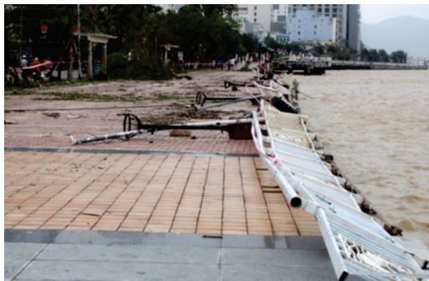
Figure 3. Typhoon Nari struck down the row railing on Bach Dang Street
