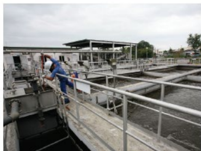
Taguig septage treatment plant (CAS)
