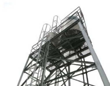
Tank for reuse of treated wastewater
