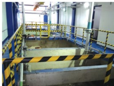
Sequential batch reactor in Project 7 WWTP
