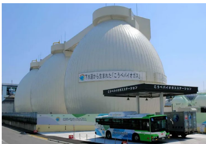
Higashinada Wastewater Treatment Plant in Kobe, Japan. Biogas from this WWTP fuels vehicles. (Photo by Japan Sanitation Consortium)
