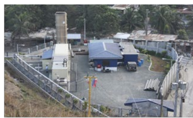
Waste to energy facility at a landfill
