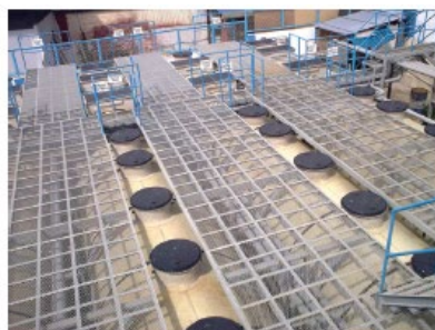
Paco WWTP using Johkasou tanks and moving bed biofilm reactor
