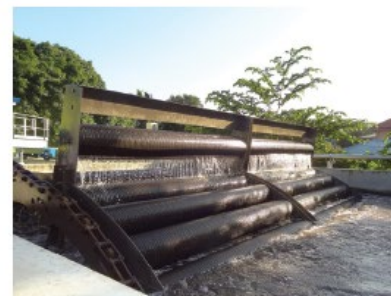
Tandang Sora WWTP using STM Aerotor
