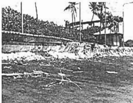
Photo 22. Beach erosion in Padang Galak.
