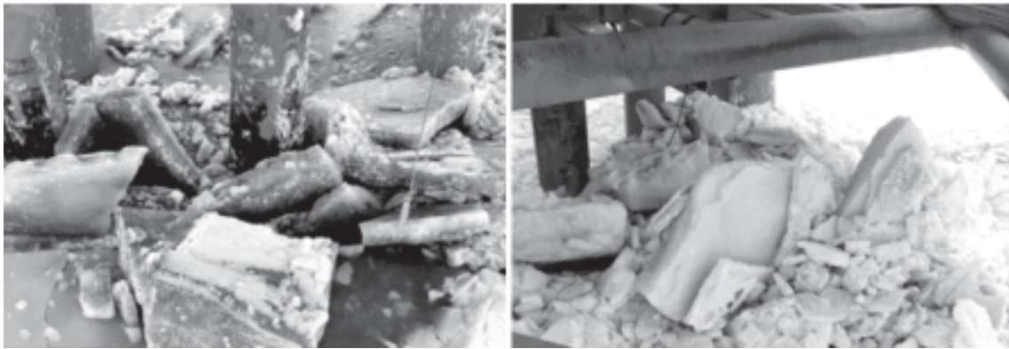
Figure 50. Maritime Engineering Structure Damaged by Sea Ice.
