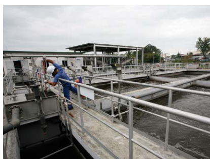
Taguig septage treatment plant
