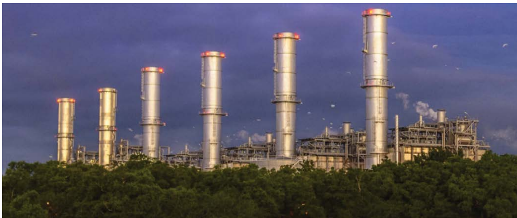
Natural gas power plant in Batangas. (Photo by First Gen)
