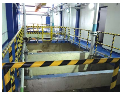
Sequential batch reactor in Project 7 WWTP
