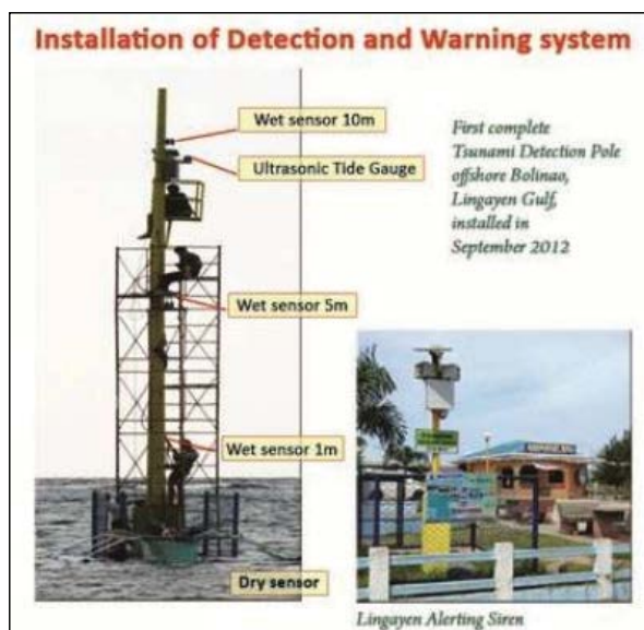
Figure 17.11: The Tsunami Early Warning System (TEWS) made Out of the Dry, Wet and Ultrasonic Sensors.
