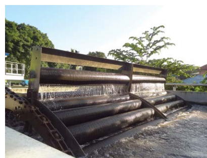
Tandang Sora WWTP using STM Aerotor (Photos by M. Ebarvia)
