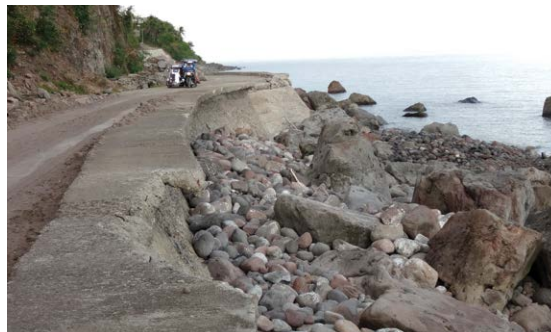
Destroyed seawall due to typhoon. (Photo by M. Ebarvia)
