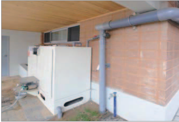
Figure 46. Changwon YMCA rainwater bank (Rainwater saving facility)
