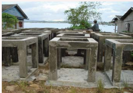
Molded blocks of concrete are left to stand for a month before deployment to avoid any negative effects of concrete on biodiversity.
